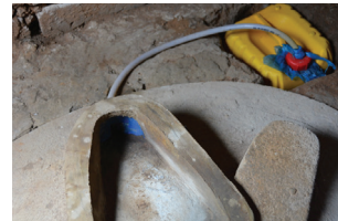
An Akasuga ecological latrine system.
